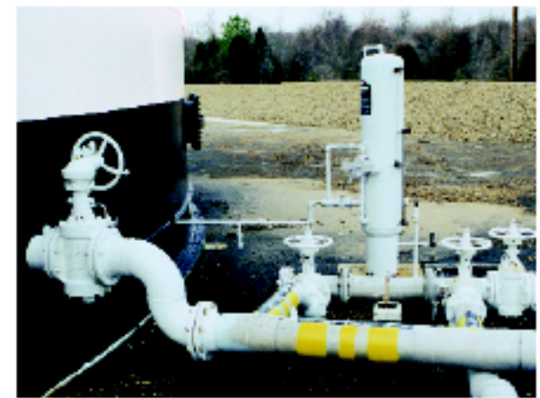
Tank-Side Isolation Maintains Product Integrity
