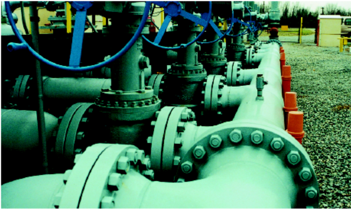
Contamination is Avoided in Multi-Products Manifolds
